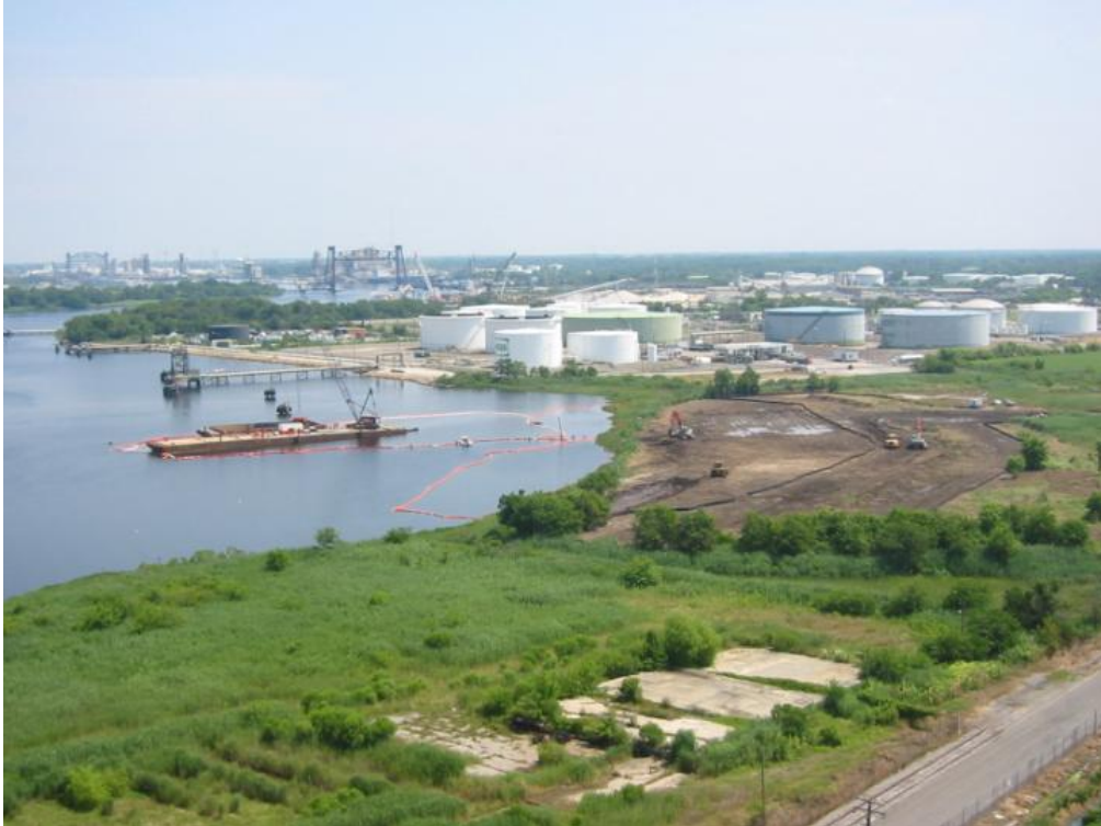
Figure 1. An overview of the Money Point dredging site on the morning of June 9, 2009. The dredge crane and barge are inside the orange oil boom/sediment curtain and the VIMS sampling vessel is outside the boom collecting water samples. Work on the constructed wetland is also visible.
