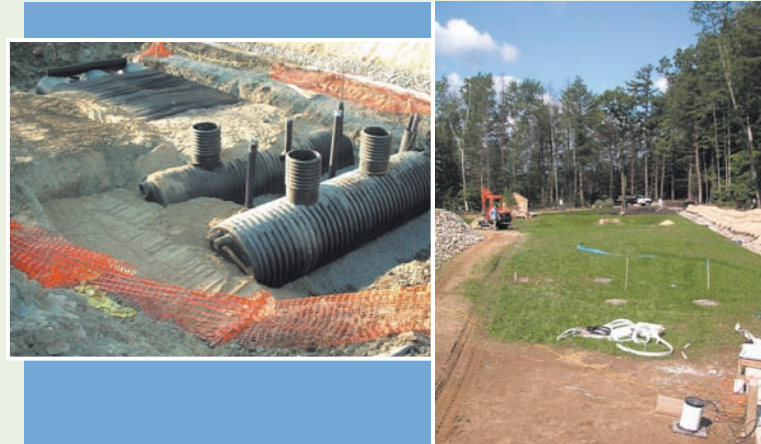
The ADS treatment system during [left] and after installation [right]. Stormwater is pretreated for sediment and floatables in the black HDPE pipes, and then flows into the adjacent storage infiltration unit, where a sandy subbase is critical to pollutant removal.
